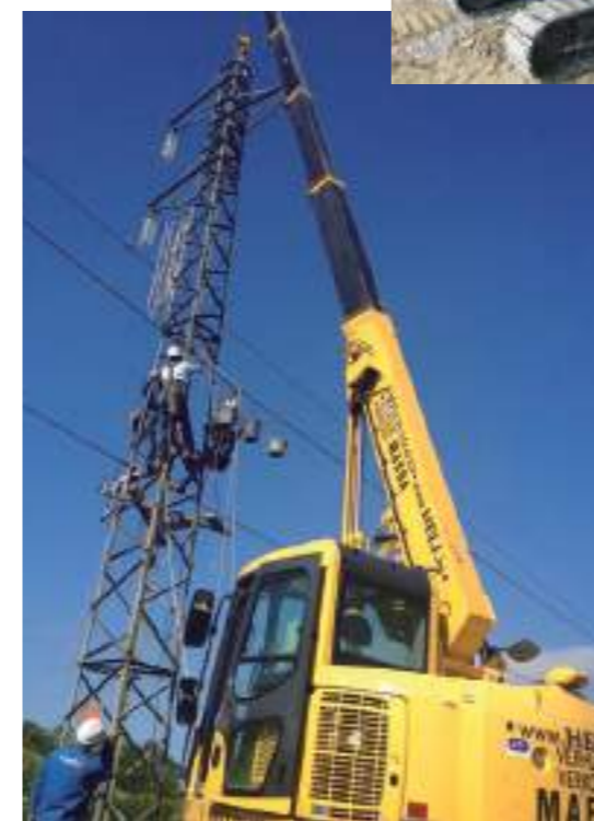
LC1385 Steel Tower
