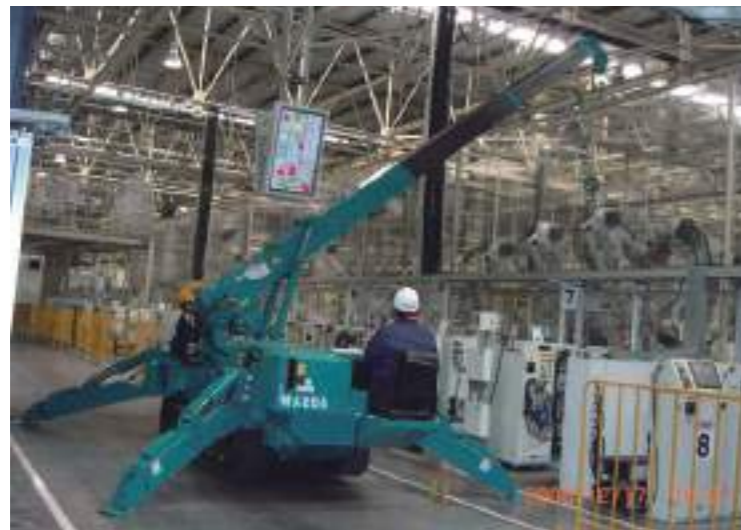
MC305C Maintenance In Factory
