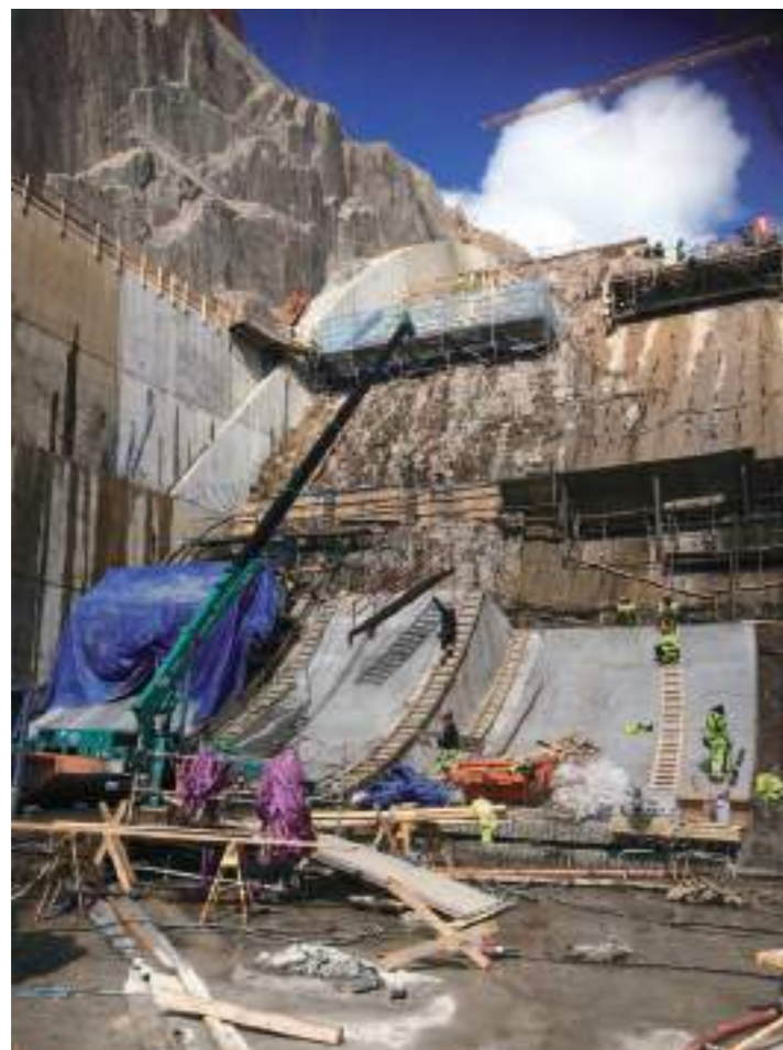
MC405C Power Plant Sweden
