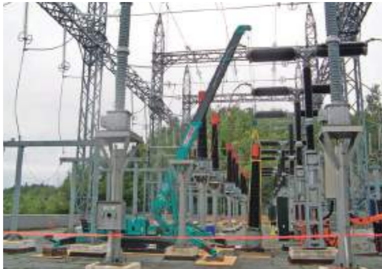
MC405C Power Station Quebec
